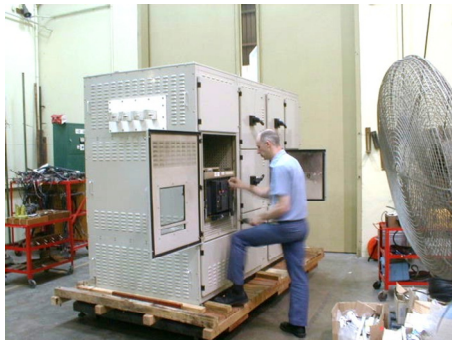
4.9 A testing engineer performing mechanical operation test.
