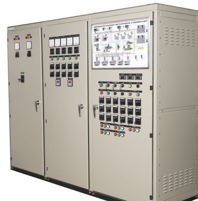
Mechanical Switchboard (Air-Con)
