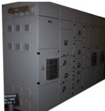
Motor control center
